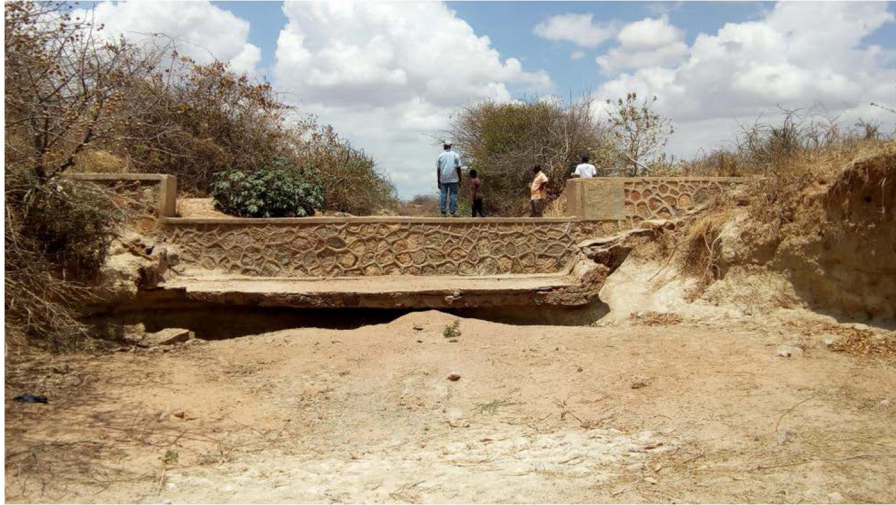
FIGURE 4 | Mshikamano sand dam near Dodoma, Tanzania exhibiting significant erosion of the apron and left streambank. Photograph taken while looking upstream during the dry season. Photo credit: J. A. Eisma.
