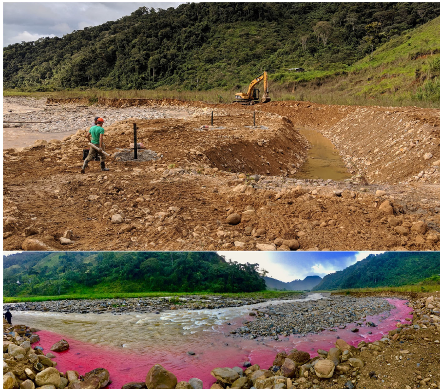
FIGURE 2 | Top: Picture of completed lateral channel oriented parallel to flow (away from camera). Rio Nambija forms the left boundary of the gravel bar, the lateral channel forms the right boundary. Three piezometers are visible in the image, with piezometers A1 and A2 in the background, piezometer B in the foreground. Bottom: Panoramic photo of tracer plume in Rio Nambija during the tracer test. The source pool is immediately below the person shown on the left side, with river flow from left to right. Lead author shown for scale. Photo credit: Samuel Lopez.
