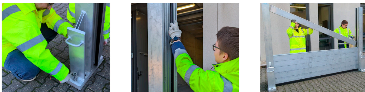
FIGURE 2 Example work steps during the construction of the MFPU: (A) Assembly of the column on the anchor plate, (B) Lubrication of the column to allow a smooth insertion of dam beams, (C) Insertion of a dam beam.
