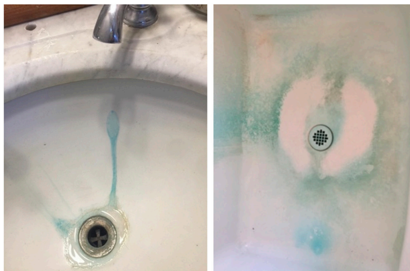
FIGURE 1 Blue-green stains due to copper contamination of water is seen on the actual sinks from the home.
