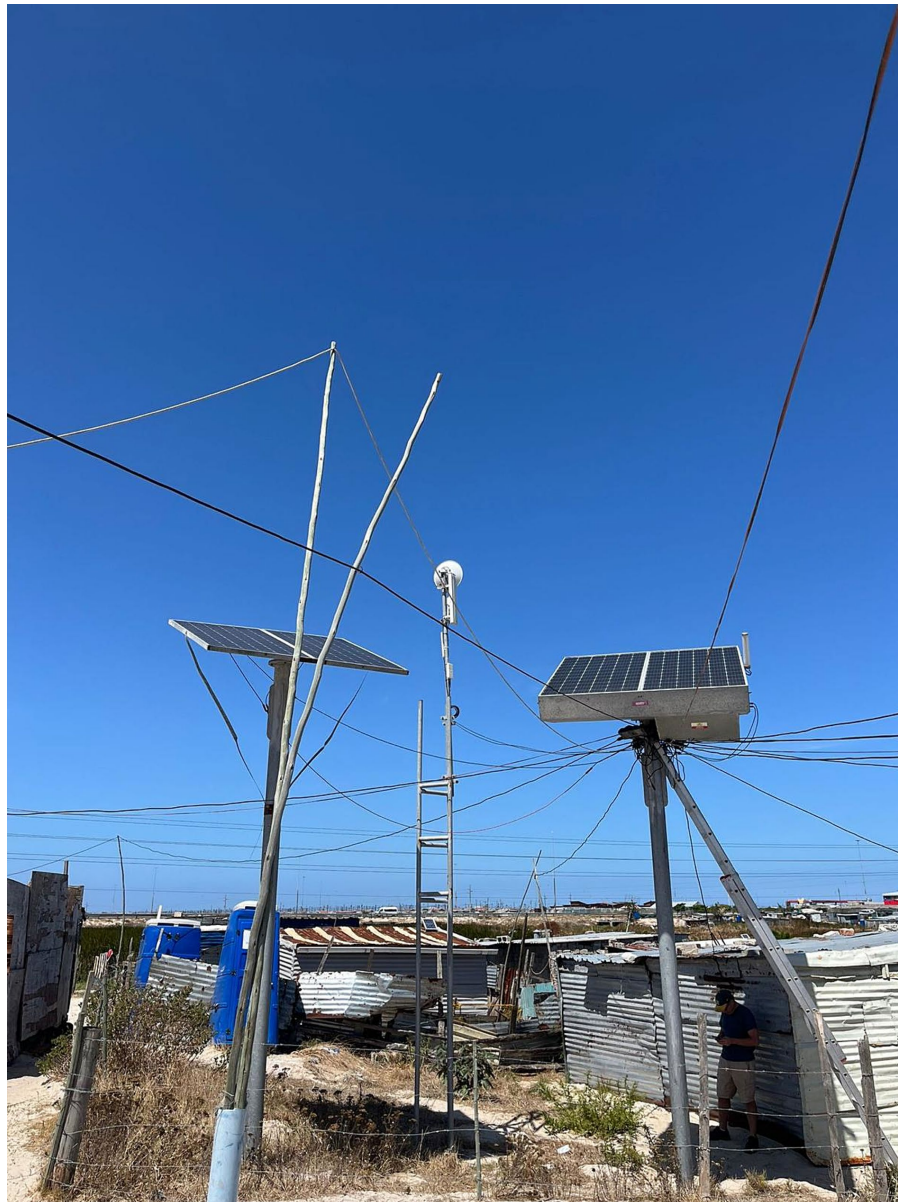
FIGURE 3 Solar towers installed in Qandu Qandu, Cape Town (source: Authors).
