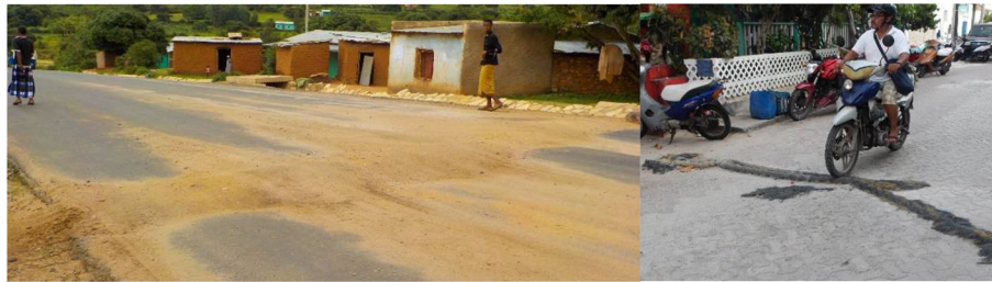
FIGURE 2 | Speed humps installed by the community: a dirt speed hump in Africa and a rope speed hump in Latin America (Source: photos by the author).
