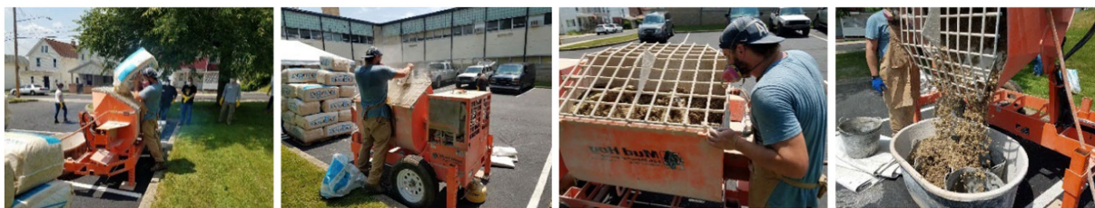
FIGURE 6 Mixing hemp hurd, lime, and water to make hempcrete for cast-in-place demonstration by Americhanvre Inc.
