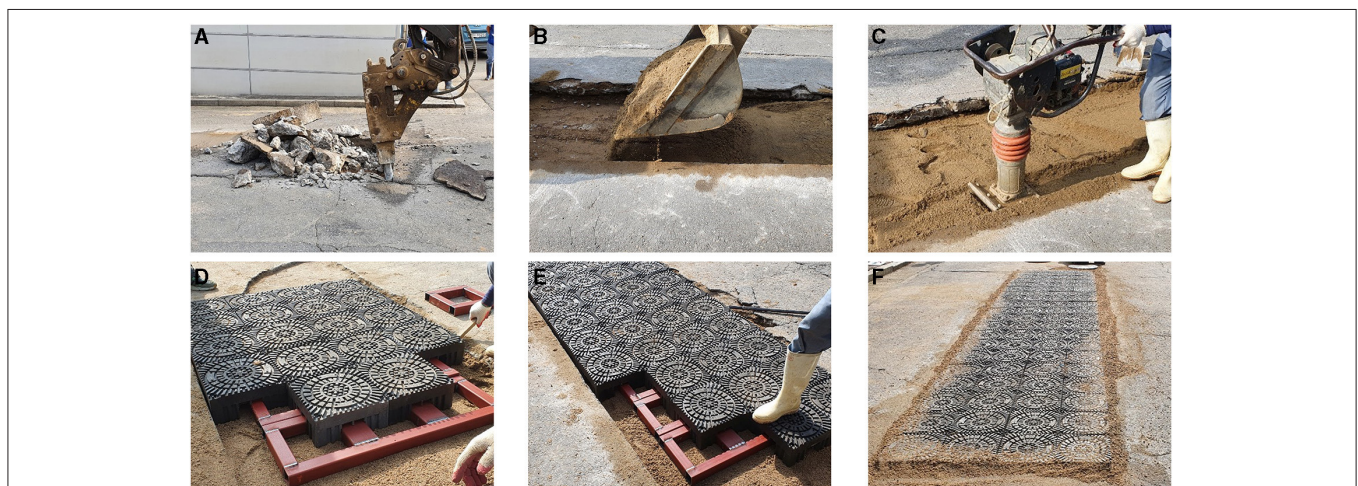
FIGURE 4 | Construction of the field test for TPB application: (A) excavation, (B) refilling, (C) compaction, (D) initiation of TPB construction, (E) TPB construction expansion, and (F) TPB construction completion.
