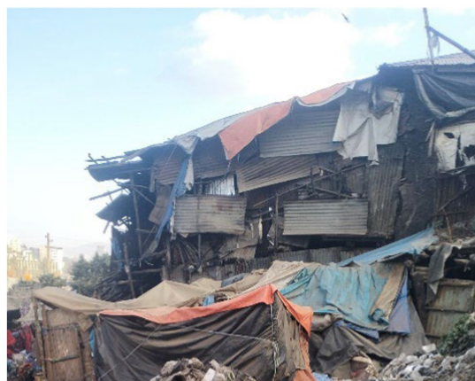
FIGURE 12 Crime Zones. Addis Ababa, Ethiopia, December 2023. These houses are rented to hide khat and other drugs, such as cocaine. They are also houses where fraudsters fabricate entirely forged documents (Image and quote credited to a mother experiencing chronic rooflessness).
