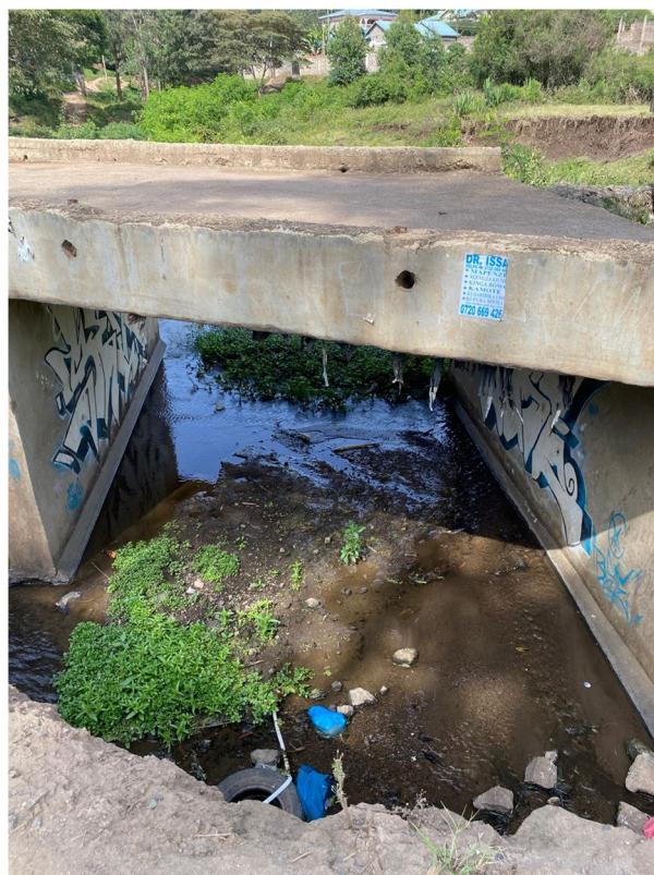
FIGURE 2 Kandisi Bridge where, in 2018, seven people drowned and 11 missing in a flash flood. The guardrail has still not been replaced. Note at this time of year the water level is very low. Authors image, February 2022.
