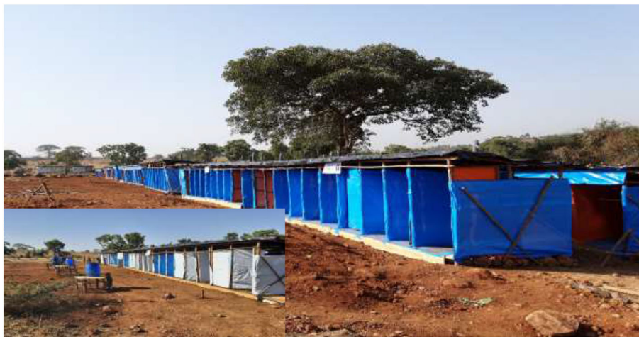
FIGURE 4 Trench latrine seats constructed in Ranch collective site, Changi, Ethiopia, November 2020 up to June 2021 ( N = 194 ).
