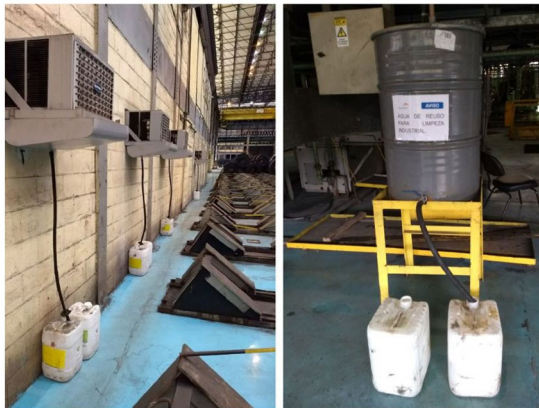
FIGURE 3 Arrangements made at the company; the installation of a system to collect the water eliminated by the air conditioning equipment, to re-use it for site cleaning.
