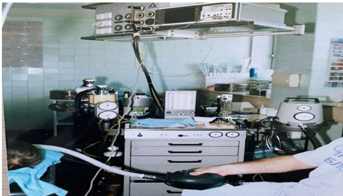
FIGURE 4 Operation Room in 2021.
