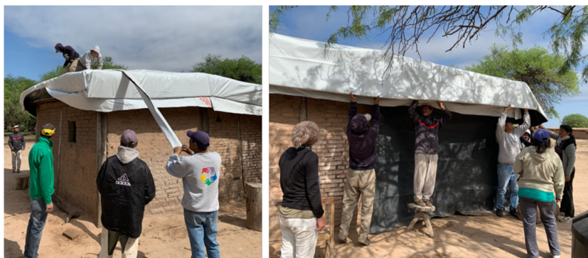
FIGURE 5 Community working groups. Pictures show community members working in groups on the improvement and waterproofing of roofs. Members worked on all houses in the location, although they do not lived in those houses, showing it was a communitarian and individual work.
