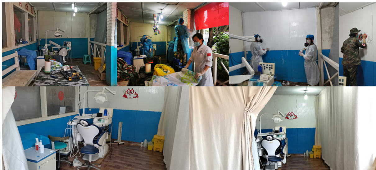
FIGURE 1 Renovation of dental clinic. Original condition. Refurbishment, brush the wall, painting, decoration completed. Outside view.
