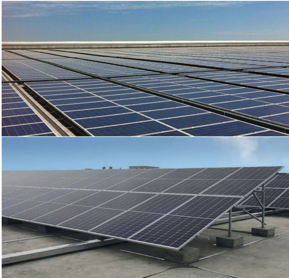
FIGURE 2 Real view of low-voltage distributed PVPP.
