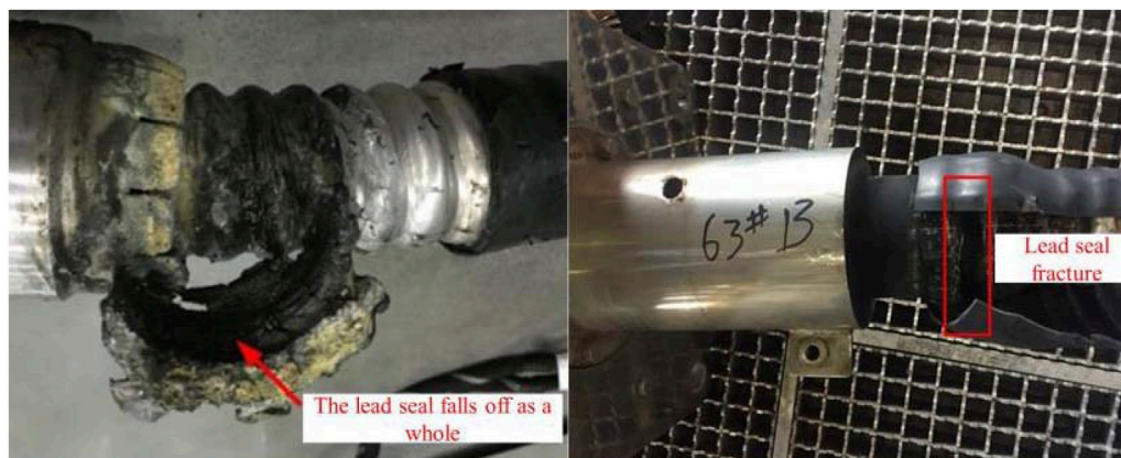
FIGURE 9 High-voltage cable lead seal failures.
