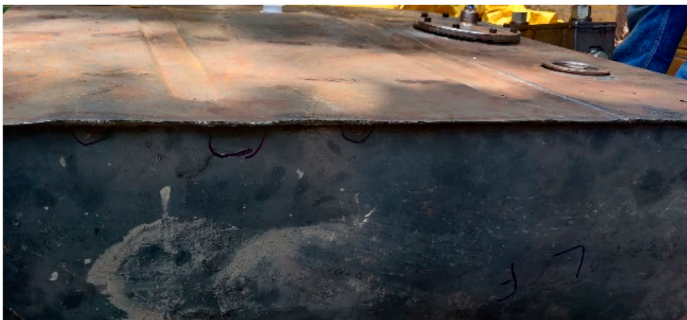
FIGURE 13 Deformed Tank under Pressure load.
