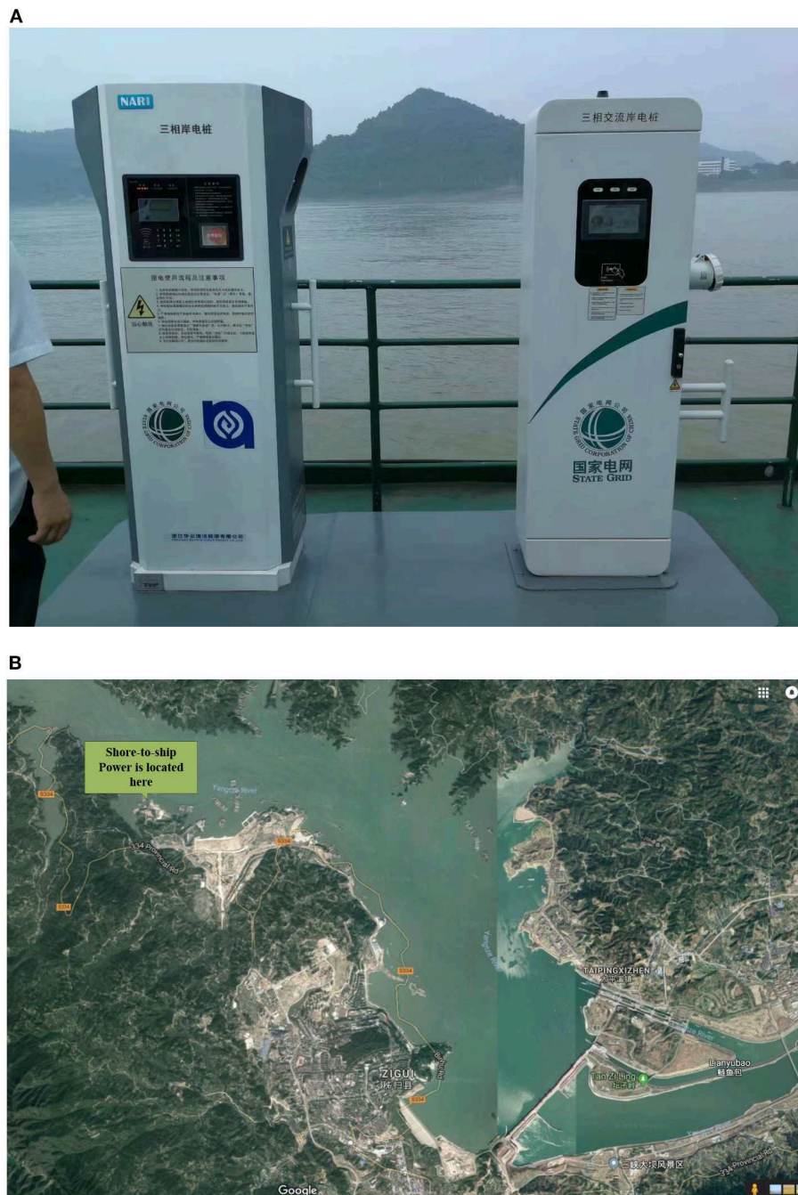
FIGURE 1 | Shore-to-ship power charging piles (China State Grid Corporation) and a map of their location beside the Yangtze River. (A) Shore-to-ship power charging piles set up by China State Grid Corporation with no cable lifting device and connection system. (B) The shore-to-ship power charging piles are located on the upper left bank of the Yangtze River Three Gorges Dam.
