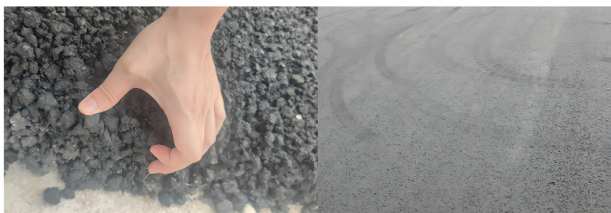
FIGURE 1 Loose and rutted new asphalt pavement.
