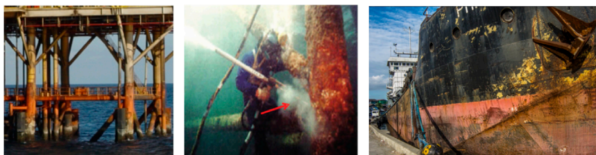
FIGURE 1 Corrosion phenomena of different marine structures.
