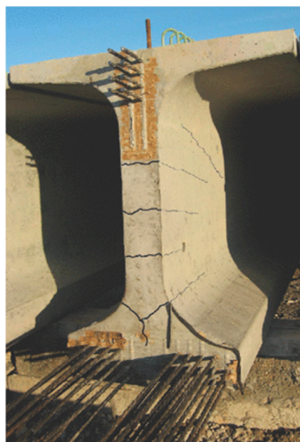
FIGURE 1 End zone cracks in a precast prestressed concrete beam (derived from Okumus and Oliva, 2013).
