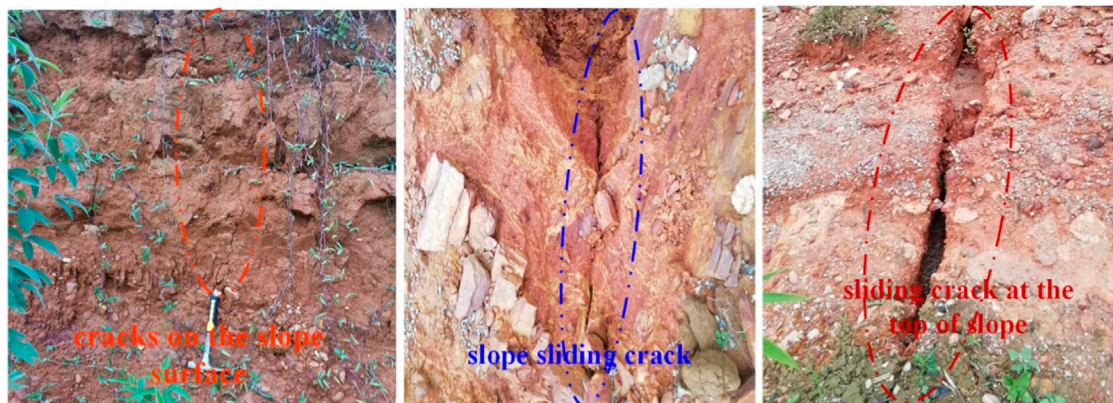
FIGURE 2 Different cracks in the slope caused by seepage after rainstorm.
