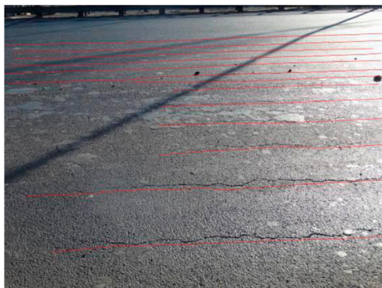
FIGURE 2 Longitudinal cracking on the asphalt pavement.
