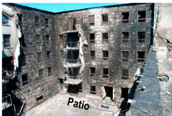
FIGURE 1 Fire consequences (Wróblewski and Stawiski, 2020).
