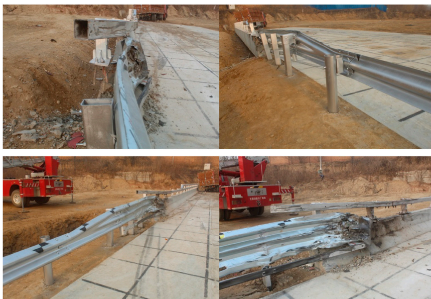
FIGURE 18 | Guardrail after the crash test.
