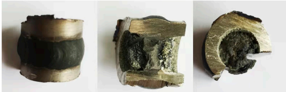
FIGURE 1 | Picture of the blockage at the welded joint of the pipe (inner diameter: 10 mm) bellow adaptor in vessel 03.
