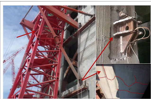
FIGURE 2 | BFJ of tower crane and cracks.
