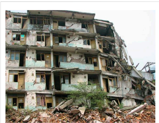
FIGURE 8 Out-of-plane collapse of walls caused by junction failure.
