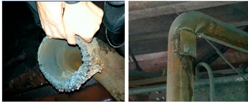
FIGURE 5 | The traditional 16 Mn steel pipeline was worn out and repaired in less than a year.
