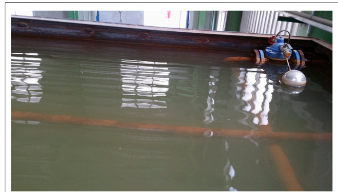
FIGURE 6 | The cistern of tailing water.
