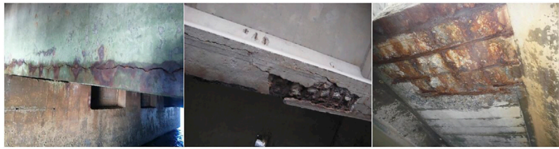
FIGURE 1 | Typical durability damage of harbor structures induced by chlorides.
