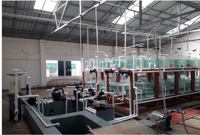
FIGURE 3 Recirculating aquaculture system (RAS) for broodstock maintenance of designer clown fish.
