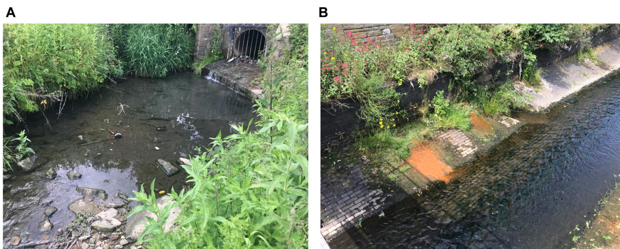
FIGURE 10 Discoloured and polluted waterbodies identified by the community group (FoBB) and community champion. These two sites ((A) shows site 1 and (B) shows site 4) were identified as possible CWQM locations (see mapped locations in Figure 7).
