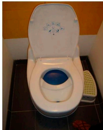
B Dry separation toilets in the apartments.
