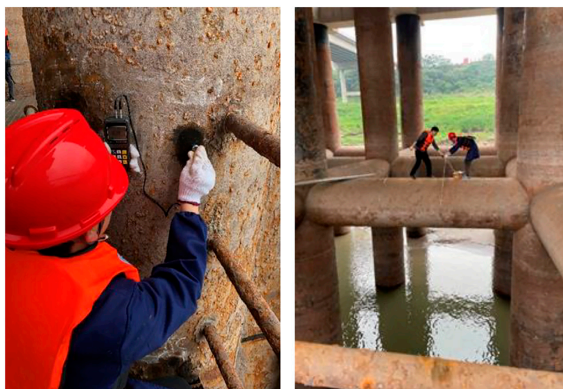
FIGURE 9 Corrosion results for steel components of a certain wharf tested in field.
