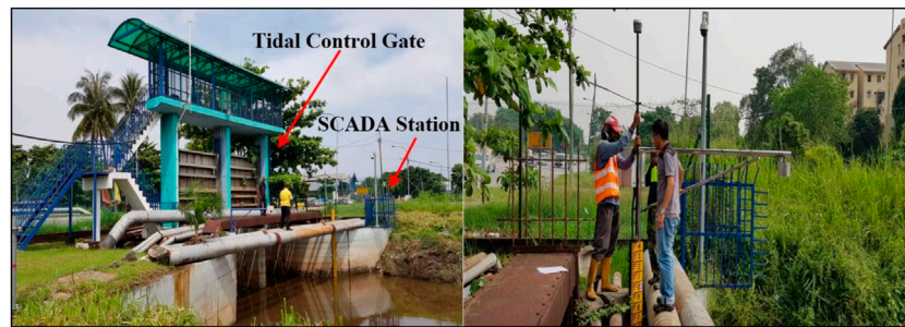
FIGURE 2 Tidal control gate and SCADA system on the Aur River. (Source: At site photos).
