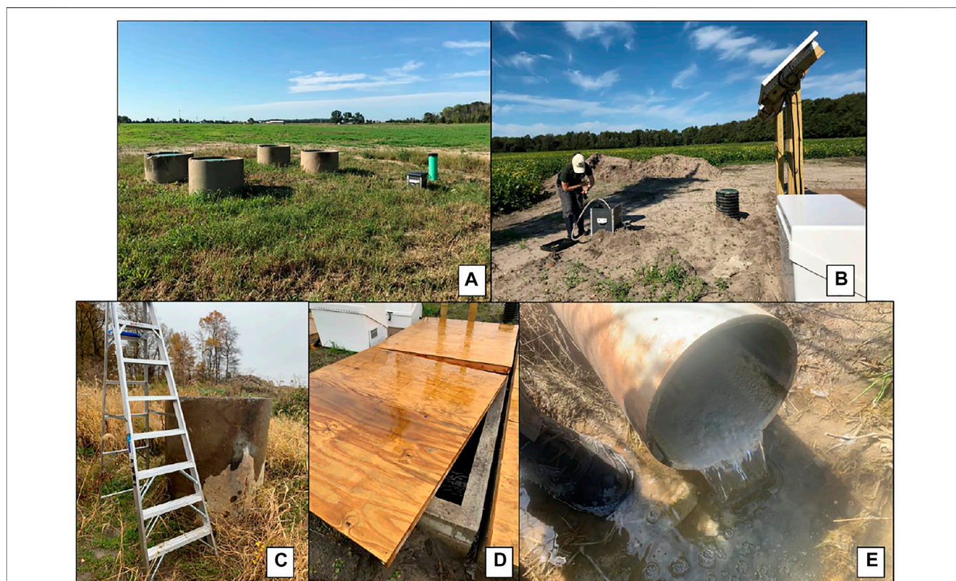
FIGURE 4 | Photos of different sampling locations. (A) Behind Mill 1 with completed iron slag filters in place. The green tube (far right) is an inflow sampling port that was installed only at this location. Access ports (for cement upright tubes) are for two slag filter basins (considered to be one slag filter site) that receive tile drain water from the adjoining field (in background) and are used to sample outflow. (B) Sampling via a hand pump siphon to sample from a below-ground control box (inflow) at Fillmore Flex; Oak Grove 2 has a similar constructed inflow access (not shown). (C) Slag filter outflow access point for Oak Grove 2, which required a ladder to remove the large plastic cap to sample outflow water. (D) Slag filter outflow access point at Fillmore Flex, which is covered with large plywood lids. (E) Outflow pipe at Behind Mill 1 directly after installation. Photo credit: Maggie Oudsema.
