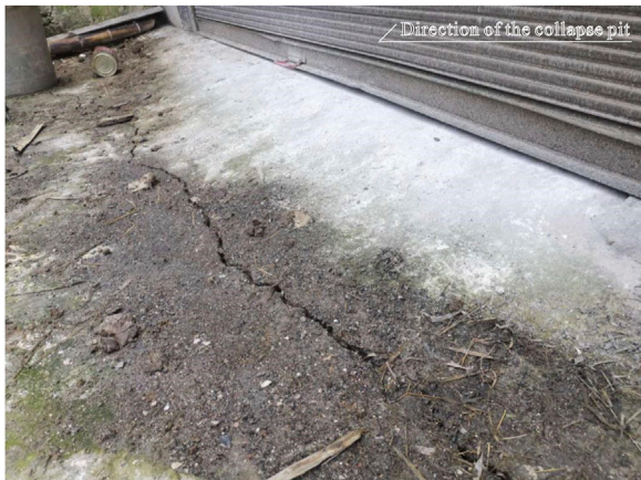
FIGURE 2 Tensile cracks in the garage of house No. 3.
