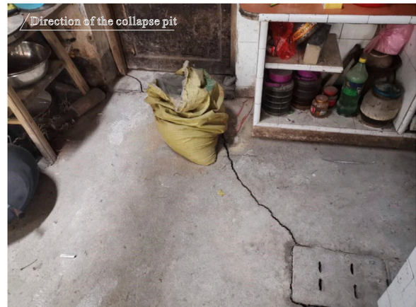
FIGURE 3 Tensile cracks in house No. 3.
