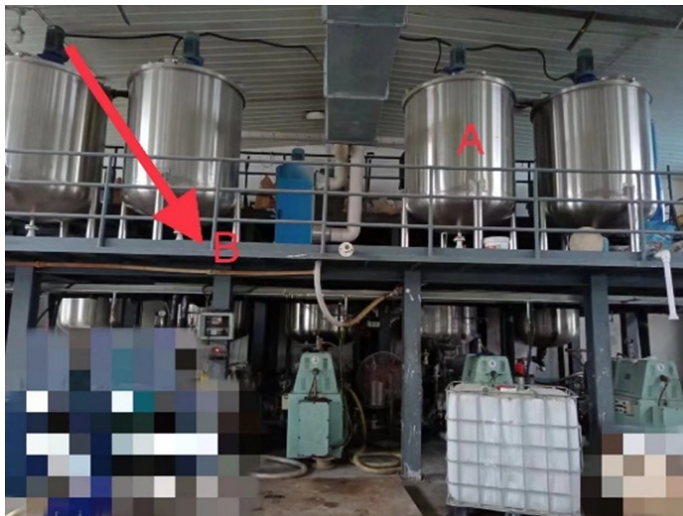
FIGURE 1 Work site environment. (Part A) Is the tank, which built up pressure and the circulation line ruptured; (Part B) Part is the blower, which caused the feed port to be blocked.
