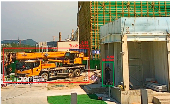
FIGURE 9 Real-time detection of construction workers and machinery for CO 2 emission estimation during substation construction.
