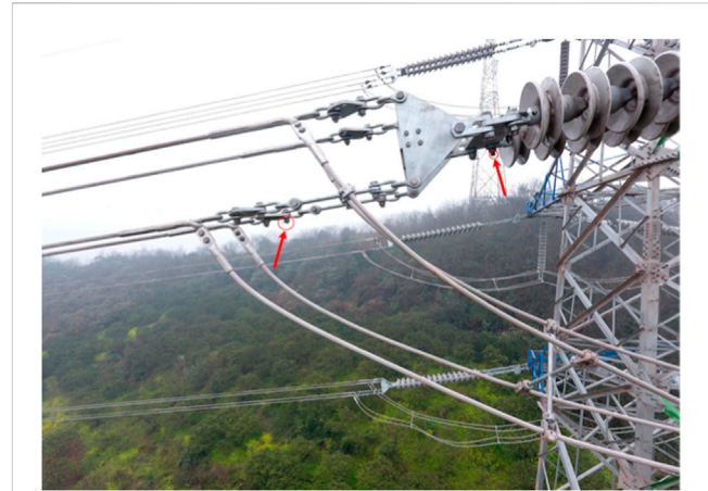
FIGURE 1 Transmission line bolt defects.
