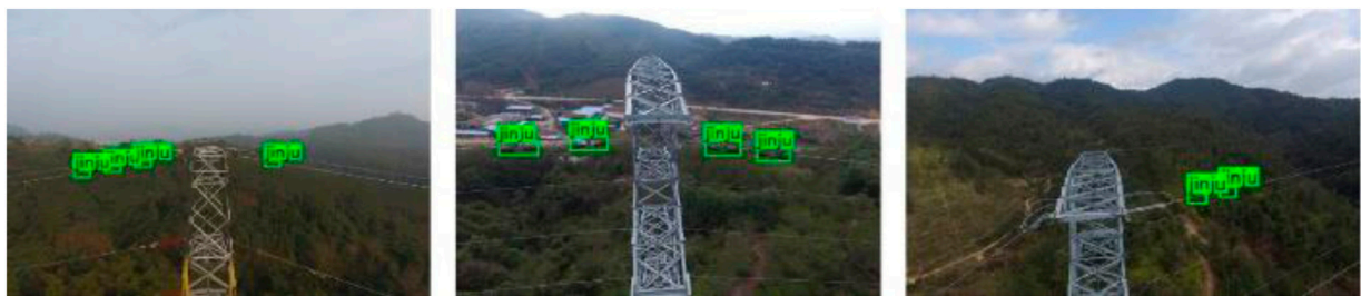
FIGURE 6 Example of fitting defects.
