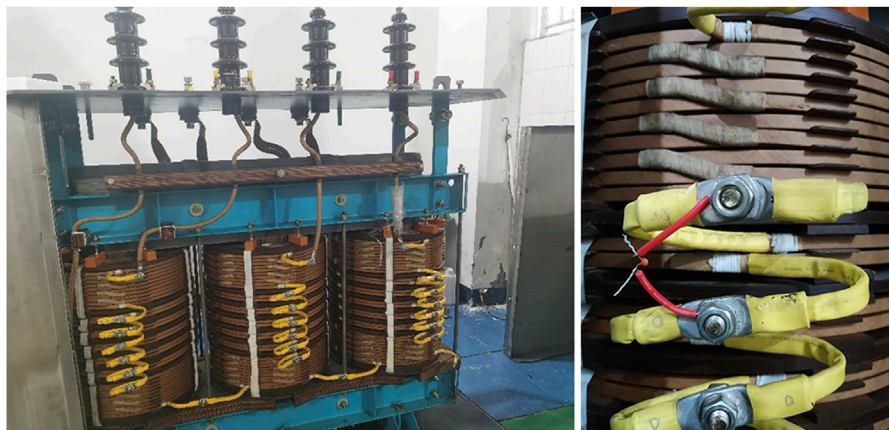
FIGURE 8 The actual photographic of transformer and the DSV fault simulation real-taken image.
