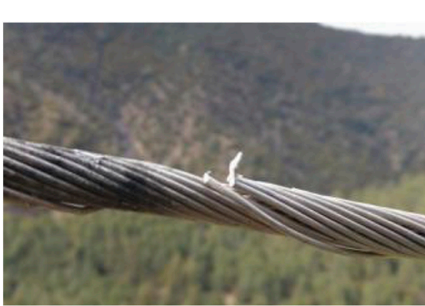
FIGURE 2 The transmission lines were broken by a lightning strike.
