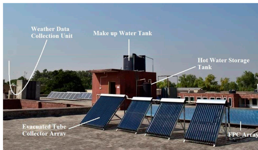
FIGURE 1 Experimental setup of solar thermal collectors.
