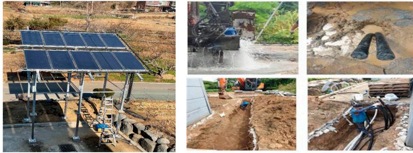
FIGURE 3 | Photovoltaic-thermal (PVT) and ground heat exchanger (GHX) installation for the polygeneration.
