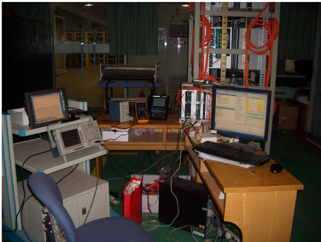
FIGURE 12 | Laboratorial 2 kV/100 kVar CMC-based STATCOM platform.
