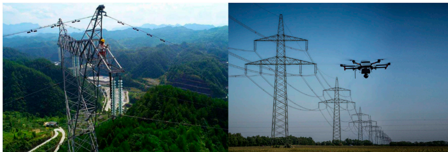
FIGURE 4 | Manual transmission line inspection and UAV inspection (Manual transmission line Inspection, 2018) (UAV transmission line Inspection, 2020).
