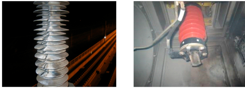
FIGURE 1 | The high-voltage equipment destroyed by the harmonic resonance.
